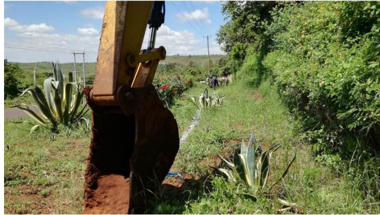
Project is starting by digging a path for the pipe to be laid
